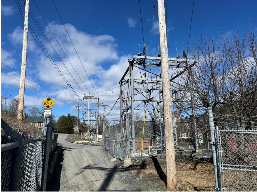
Photograph 26: Taftsville Hydroelectric Station, East Substation.
