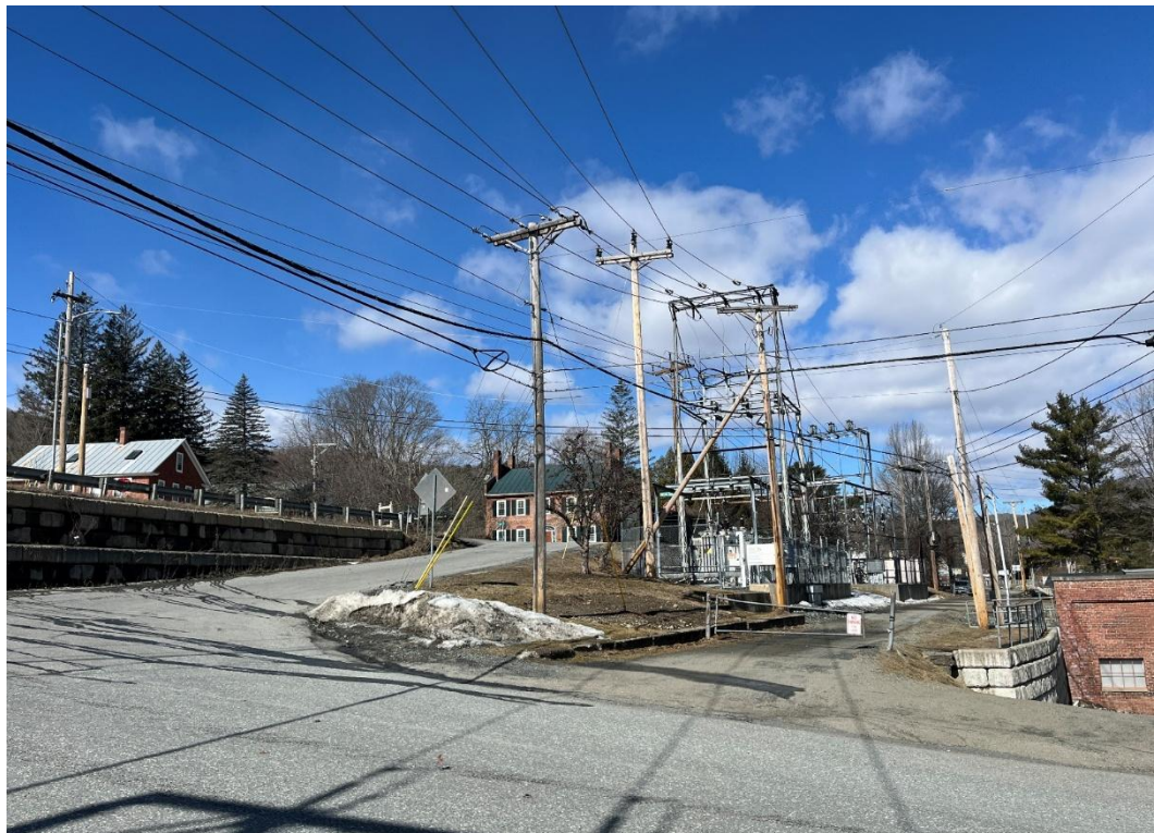
Photograph 5: Looking northwest to the distribution and west substations and hydroelectric station.
