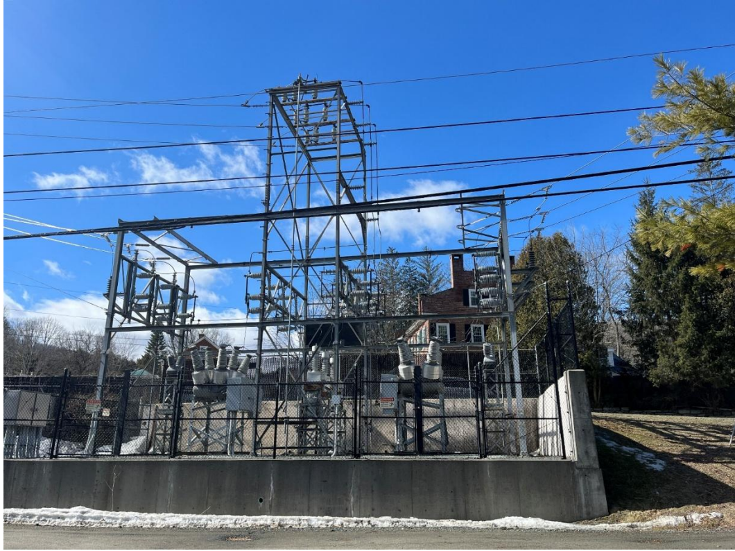
Photograph 24: Taftsville Hydroelectric Station.
