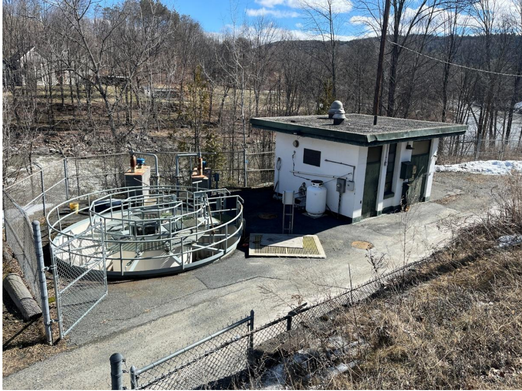
Photograph 18: Water Treatment Plant.
