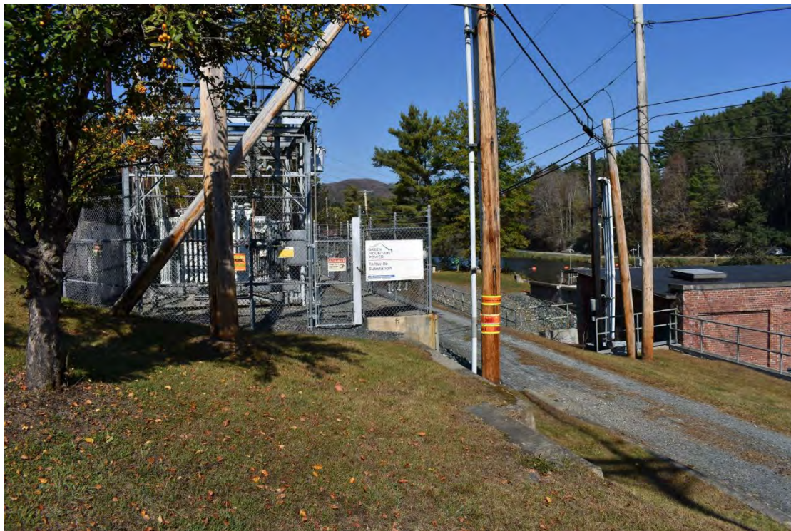
Figure 25. View west of the Transmission substation structure of the Taftsville Substation, located in the North Study Area of the GMP Taftsville Substation Relocation Project, Woodstock and Hartland, Windham County, Vermont.
