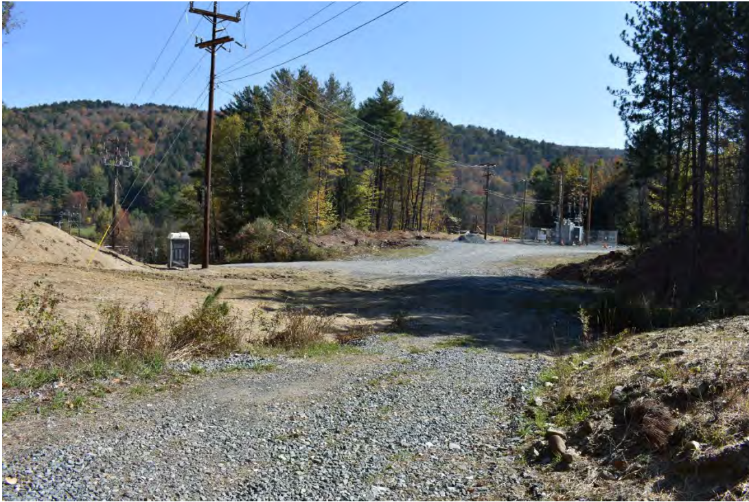
Figure 36. View south of the temporary GMP Taftsville Substation in the area of the former gravel pit in the northern portion of the South Study Area of the GMP Taftsville Substation Relocation Project, Woodstock and Hartland, Windsor County, Vermont.
