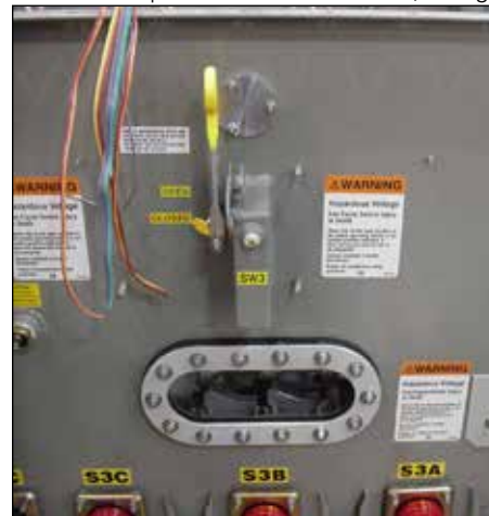
Figure 8. VFI transformer with visible break.
