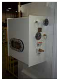
Figure 7. External visible break with gauges.
