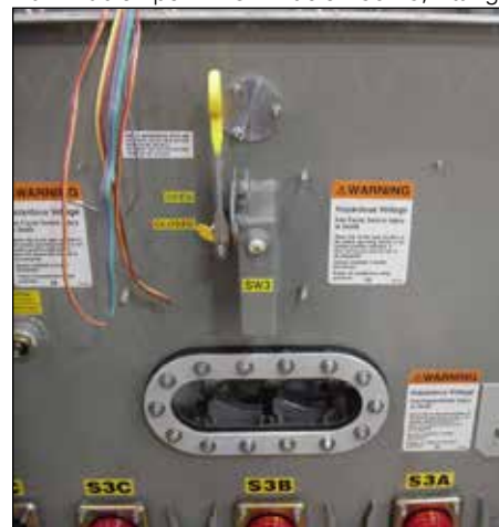
Figure 8. VFI transformer with visible break.
