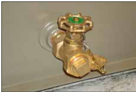
Figure 3. Drain valve with sampler.
