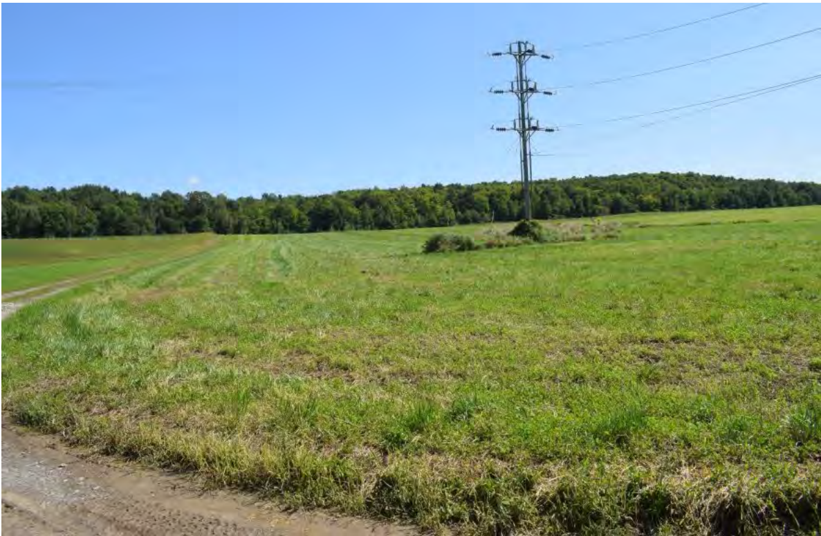
Figure 17. View east of transmission line structure to be replaced as part of the Green Mountain Power Georgia Substation Upgrade Project, Franklin County, Vermont. Note farm road that cuts through area.
