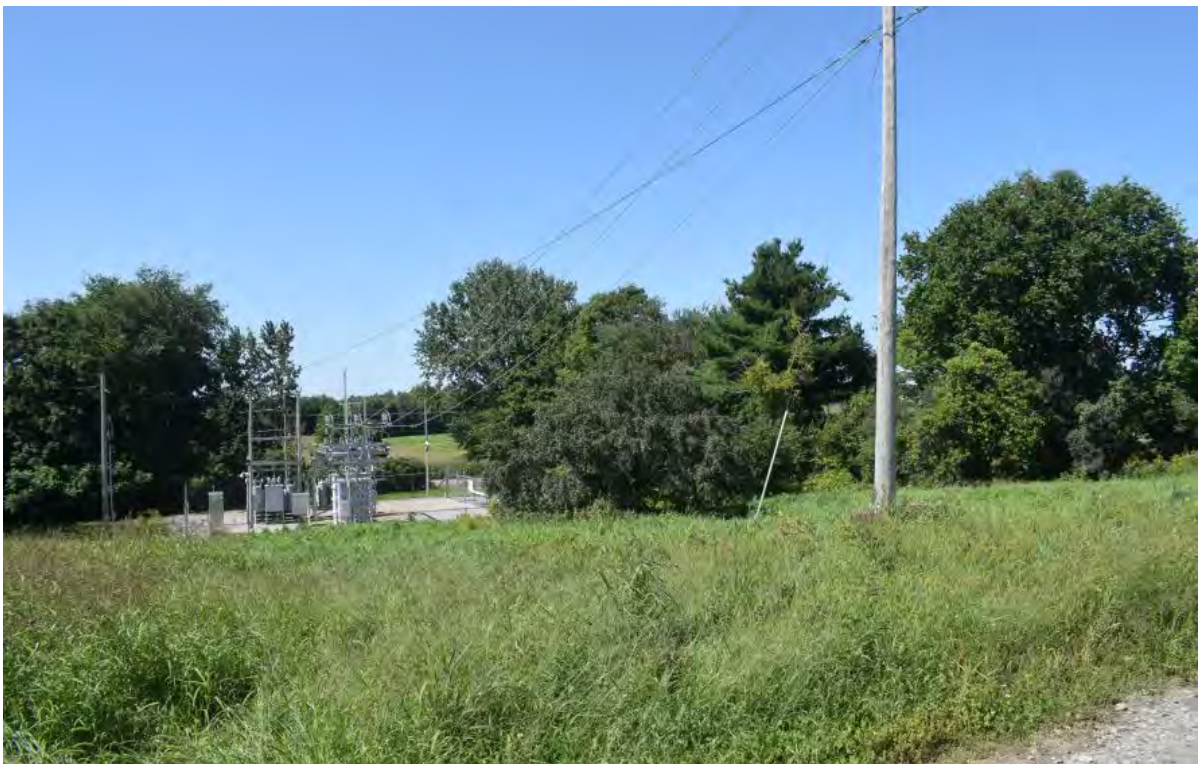
Figure 15. View west of the existing Green Mountain Power Georgia Substation Upgrade Project, Franklin County, Vermont.
