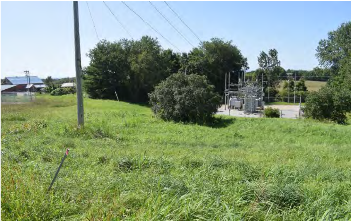
Figure 14. View west of the existing Green Mountain Power Georgia Substation Upgrade Project, Franklin County, Vermont.
