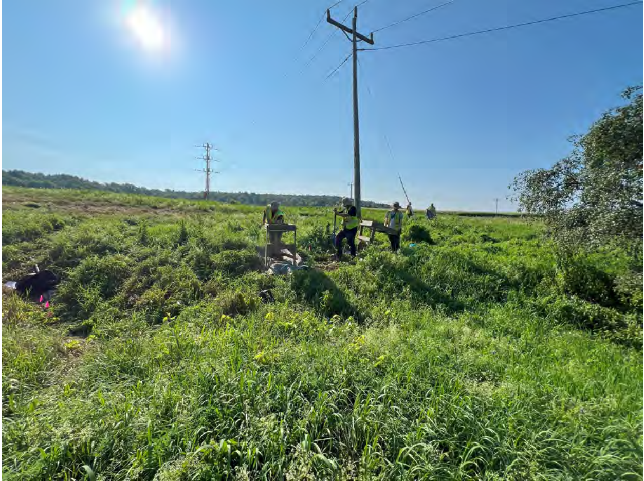
Figure 7. View southeast of the NE ARC field crew excavating test pits along Transect 5 at the proposed Green Mountain Power Georgia Substation Upgrade Project, Franklin County, Vermont.
