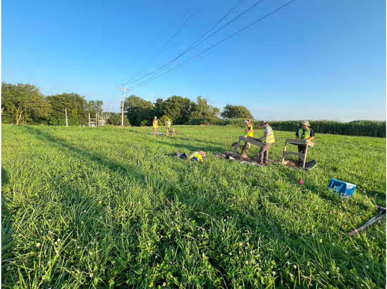
Figure 8. View west of NE ARC crew excavating along transect T6 at the proposed Green Mountain Power Georgia Substation Upgrade Project, Franklin County, Vermont. Note the GMP structures and substation.
