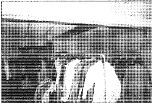
21-22. Above, Typical rear ell basement views of south room 23. Above, right, Typical rear ell basement view of north room.
