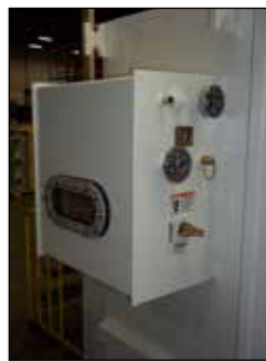
Figure 7. External visible break with gauges.
