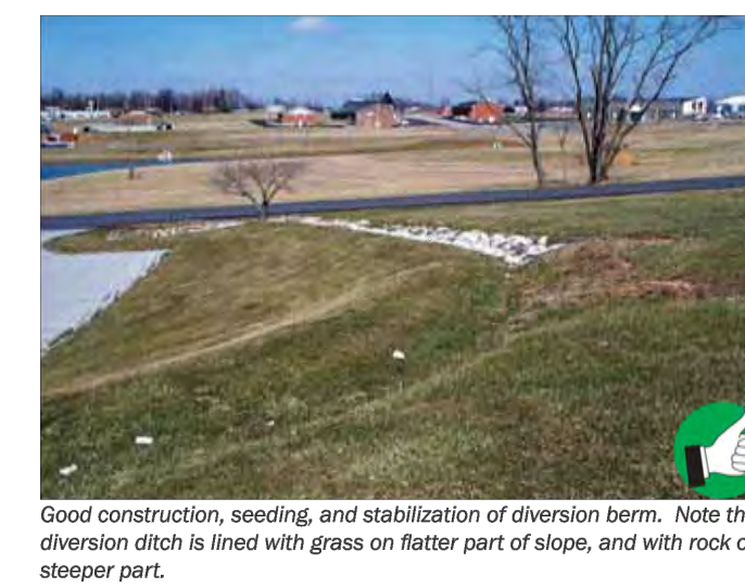
Good construction, seeding, and stabilization of diversion berm. Note that diversion ditch is lined with grass on flatter part of slope, and with rock on steeper part.
