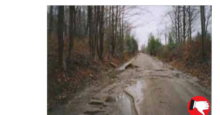
Hay bales must not be used as check dams due to their high failure rates.
