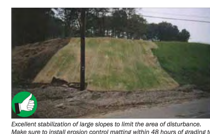
Excellent stabilization of large slopes to limit the area of disturbance. Make sure to install erosion control matting within 48 hours of grading to ensure good contact between soil and mat.
