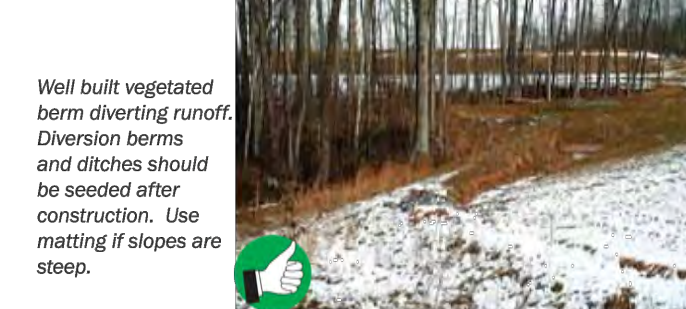
Well built vegetated berm diverting runoff. Diversion berms and ditches should be seeded after construction. Use matting if slopes are steep.
