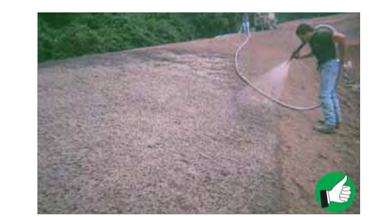
Hydroseeding exposed soil is a good option for stabilizing large areas. Hydroseed is a mixture of seed, fertilizer, water and a tackifier to hold the seed in place before it germinates.
