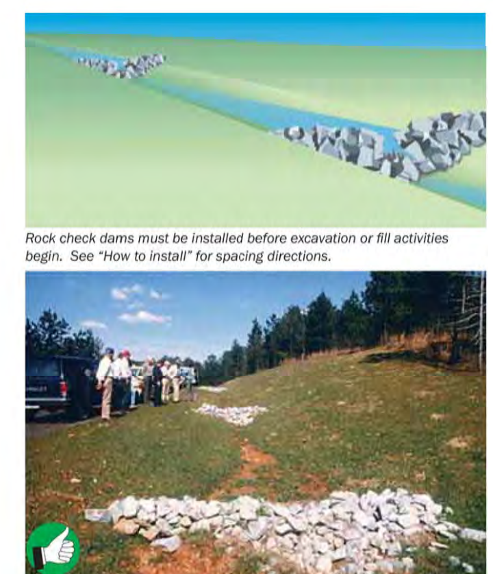
Good installation of temporary rock check dams. The check dams should extend up the sides of the banks. Middle section should be lower than the sides. Clean out sediment as it accumulates. Remove check dams after site and channel are stabilized with vegetation. Slow Down Channelized Runoff 21
