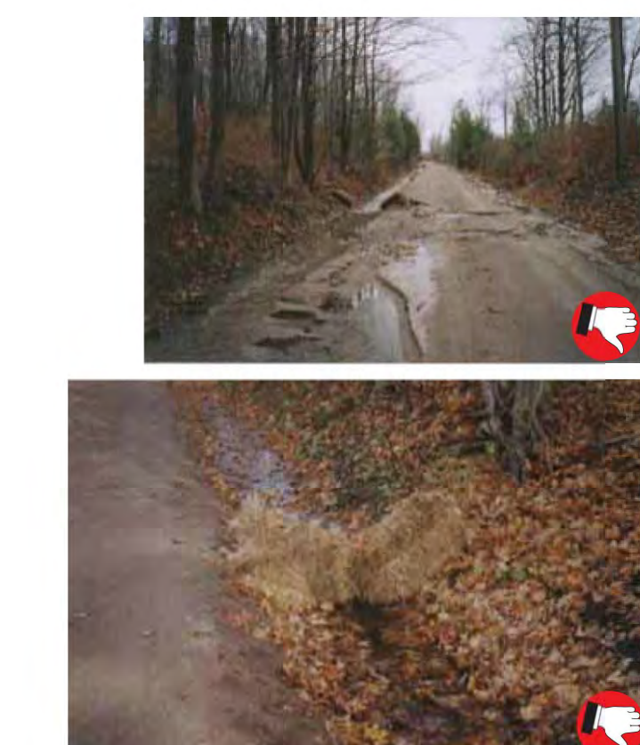
Good installation of temporary rock check dams. The check dams should extend up the sides of the banks. Middle section should be lower than the sides. Clean out sediment as it accumulates. Remove check dams after site and channel are stabilized with vegetation. Slow Down Channelized Runoff 21
