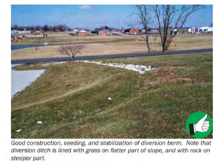
Good construction, seeding, and stabilization of diversion berm. Note that diversion ditch is lined with grass on flatter part of slope, and with rock on steeper part. 17
