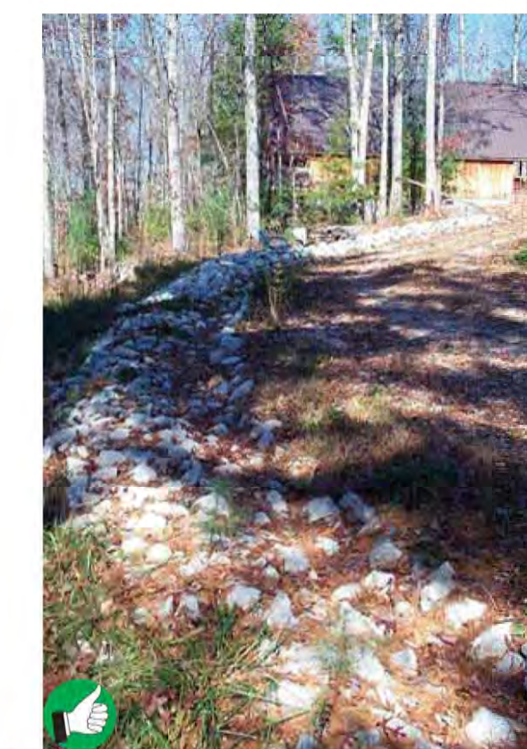
Good installation of rock-lined berm to divert rain runoff around residential construction site on steep slope near a river. Diversion ditches can be lined with grass if channel slopes are 5% or less, and with 4 inch stone if they are steeper. 18
