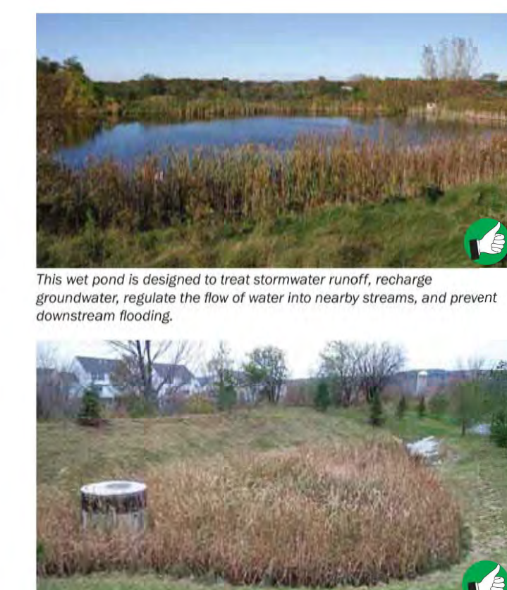
Install all permanent stormwater treatment practices before constructing any impervious surfaces on site. This stormwater wetland treats stormwater runoff from the adjacent parking lot. Construct Permanent Controls 24
