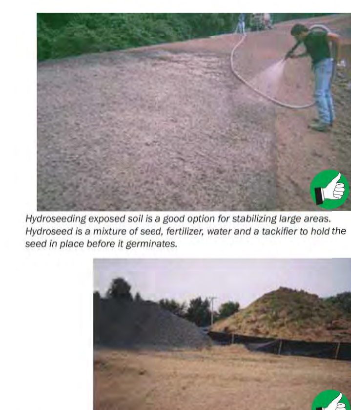
Excellent application of hay mulch. Good mulch cover and sediment barrier around soil stockpile. Stabilize Exposed Soil 28
