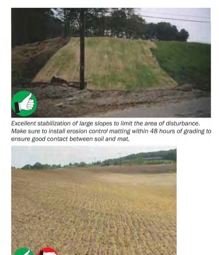
Good tracking up and down slope. Tracking slows down runoff and promotes infiltration. More mulch is needed. Stabilize Exposed Soil 27
