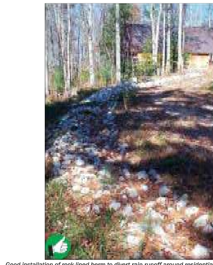
Good installation of rock-lined berm to divert rain runoff around residential construction site on steep slope near a river. Diversion ditches can be lined with grass if channel slopes are 5% or less, and with 4 inch stone if they are steeper. 18
