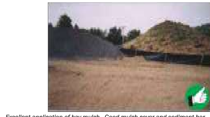
Excellent application of hay mulch. Good mulch cover and sediment barrier around soil stockpile. 28
