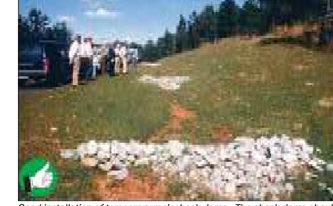
Good installation of temporary rock check dams. The check dams should extend up the sides of the banks. Middle section should be lower than the sides. Clean out sediment as it accumulates. Remove check dams after site and channel are stabilized with vegetation. 21
