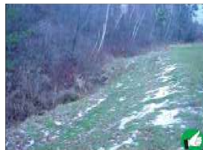
Stabilization and seeding of slopes before winter will reduce or eliminate erosion in the spring. The grass on this slope is holding the soil in place and promoting infiltration of the melting snow. 30
