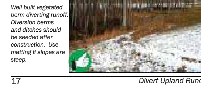
Well built vegetated berm diverting runoff. Diversion berms and ditches should be seeded after construction. Use matting if slopes are steep. 17
