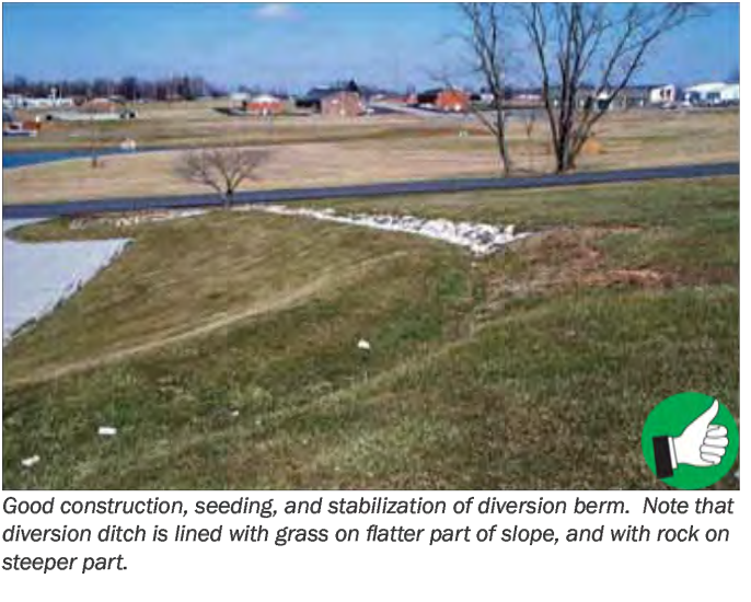
Good construction, seeding, and stabilization of diversion berm. Note that diversion ditch is lined with grass on flatter part of slope, and with rock on steeper part. 17
