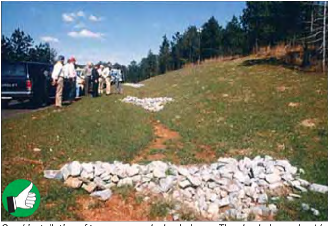
Good installation of temporary rock check dams. The check dams should extend up the sides of the banks. Middle section should be lower than the sides. Clean out sediment as it accumulates. Remove check dams after site and channel are stabilized with vegetation. Slow Down Channelized Runoff 21
