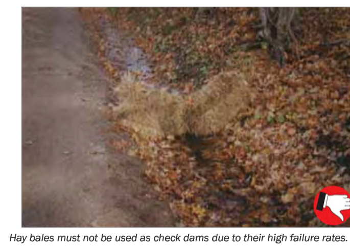
Hay bales must not be used as check dams due to their high failure rates. Good installation of temporary rock check dams. The check dams should extend up the sides of the banks. Middle section should be lower than the sides. Clean out sediment as it accumulates. Remove check dams after site and channel are stabilized with vegetation. Slow Down Channelized Runoff 22
