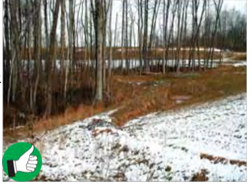
Well built vegetated berm diverting runoff. Diversion berms and ditches should be seeded after construction. Use matting if slopes are steep. 17
