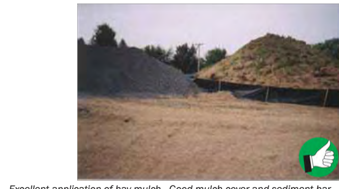
Excellent application of hay mulch. Good mulch cover and sediment barrier around soil stockpile. Stabilize Exposed Soil 28
