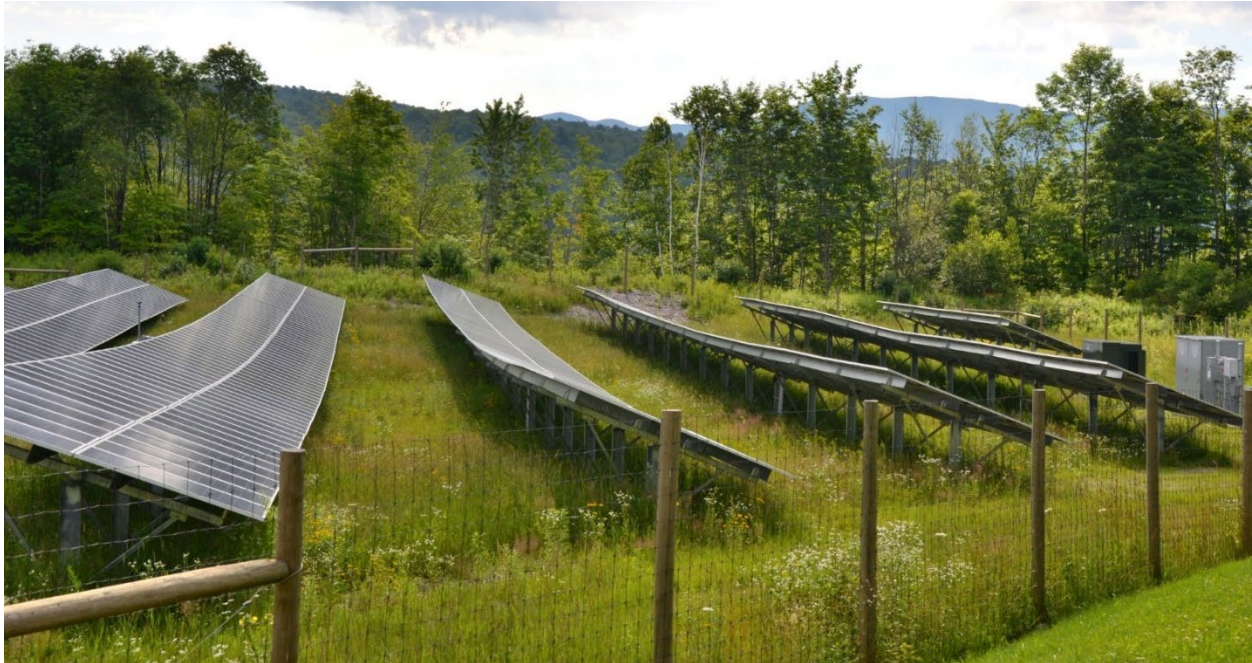
Figure 1: Example of ground-mounted fixed-tilt array racks in east-west orientation.
