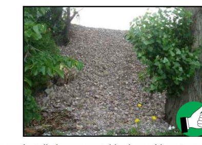
Stone rip-rap installed on an unstable slope with a stormwater outlet pipe along the slope.
