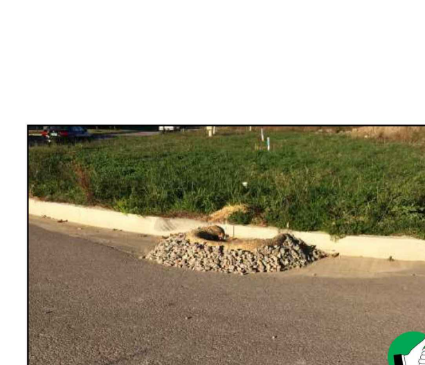
Use of stone inlet protection with the incorporation of a straw wattle in place of cinder blocks for the stone and block specification.
