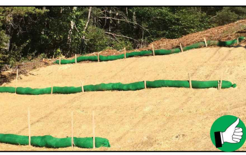
Good use of filter socks along a slope to slow runoff velocity.
