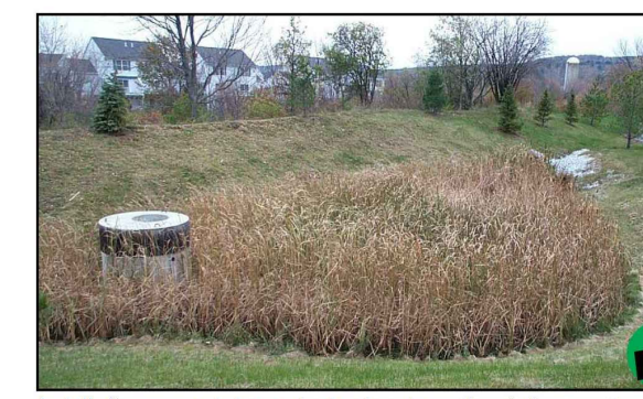
Install all permanent stormwater treatment practices before constructing any impervious surfaces on site. This stormwater wetland treats stormwater runoff from the adjacent parking lot.
