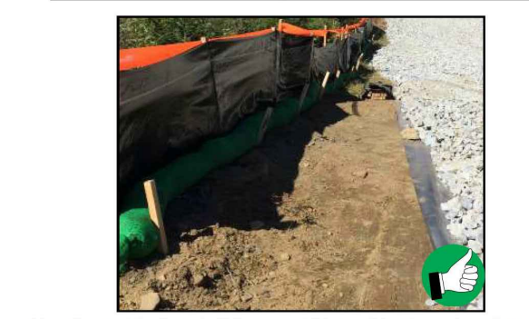
Use of a combination of silt fence and filter sock in place of reinforced silt fence for winter construction perimeter control requirements in proximity to a water resource area.
