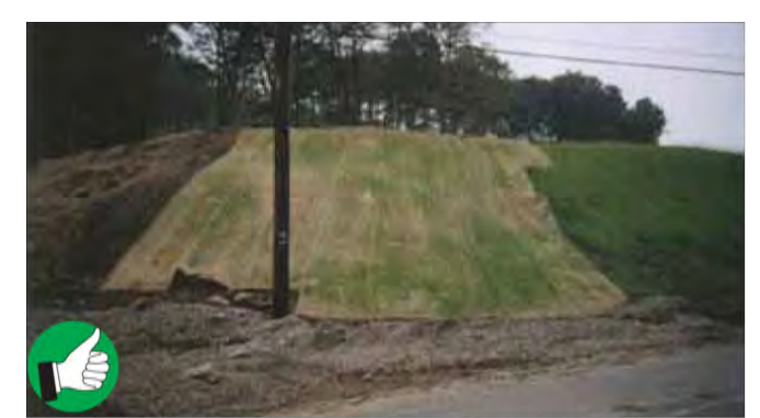
Excellent stabilization of large slopes to limit the area of disturbance. Make sure to install erosion control matting within 48 hours of grading to ensure good contact between soil and mat.
