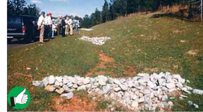
Good installation of temporary rock check dams. The check dams should extend up the sides of the banks. Middle section should be lower than the sides. Clean out sediment as it accumulates. Remove check dams after site and channel are stabilized with vegetation.
