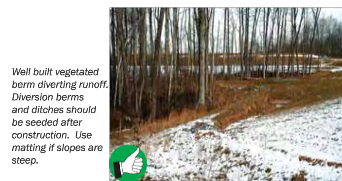
Good construction, seeding, and stabilization of diversion berm. Note that diversion ditch is lined with grass on flatter part of slope, and with rock on steeper part.
