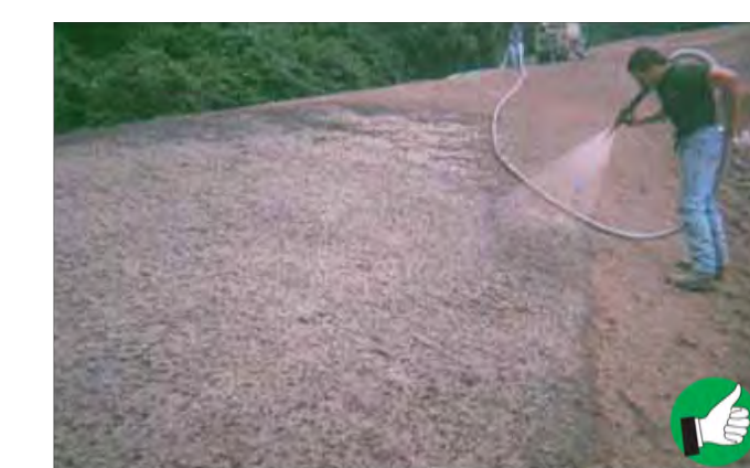
Hydroseeding exposed soil is a good option for stabilizing large areas. Hydroseed is a mixture of seed, fertilizer, water and a tackifier to hold the seed in place before it germinates.
