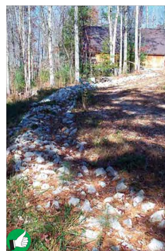
Good installation of rock-lined berm to divert rain runoff around residential construction site on steep slope near a river. Diversion ditches can be lined with grass if channel slopes are 5% or less, and with 4 inch stone if they are steeper.
