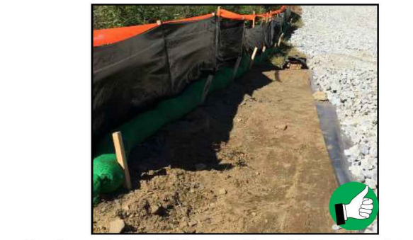
Use of a combination of silt fence and filter sock in place of reinforced silt fence for winter construction perimeter control requirements in proximity to a water resource area.
