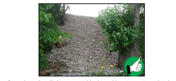
Stone rip-rap installed on an unstable slope with a stormwater outlet pipe along the slope.
