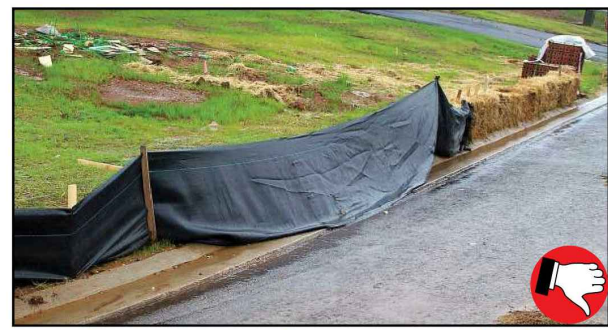
Poor installation of silt fencing. Silt fence must be trenched in along bottom. Hay bales are not approved as sediment barriers.
