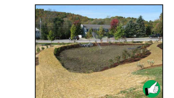
Infiltrating stormwater practices such as this bioretention system should be kept offline until the drainage area has been fully stabilized.
