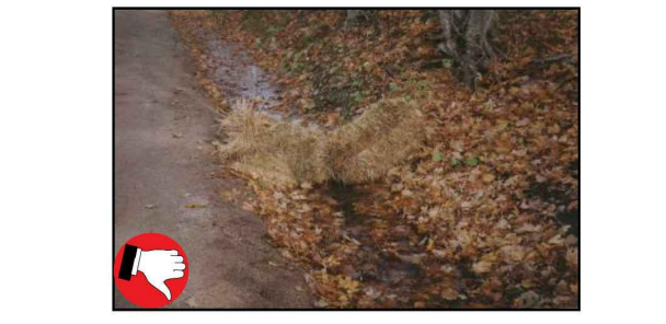
Hay bales must not be used as check dams due to their high failure rates.
