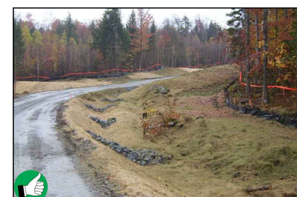
Good installation of rock check dams. The check dams should extend up the sides of the banks. Middle section should be lower than the sides. Clean out sediment as it accumulates.
