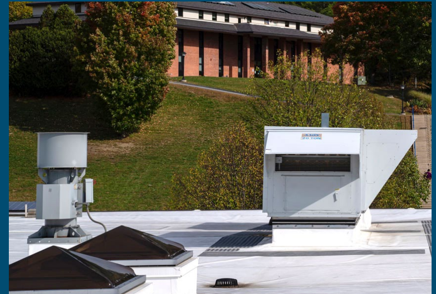
FLM-enrolled HVAC infrastructure at Landmark College
