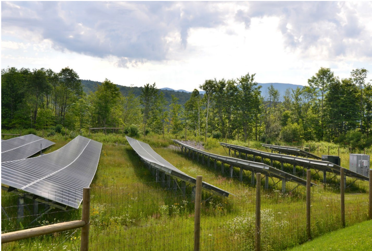
Figure 1: Example of fixed-tilt racking units with dual portrait panels.
