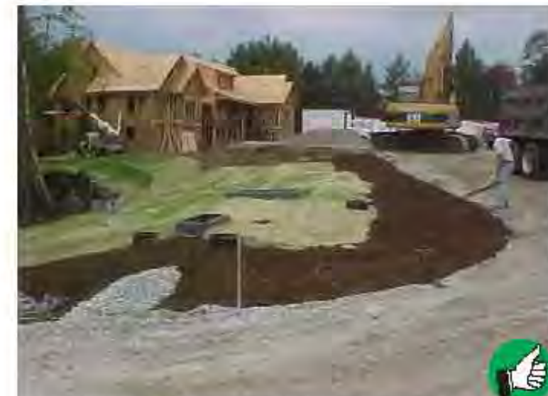
Within 48 hours of final grading, erosion control matting and mulch have been applied.
