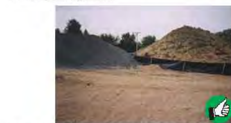
Excellent application of hay mulch. Good mulch cover and sediment barrier around soil stockpile.
