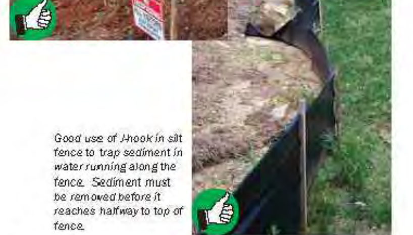
Good use of hook in silt fence to trap sediment in water running along the fence. Sediment must be removed before it reaches halfway to top of fence.
