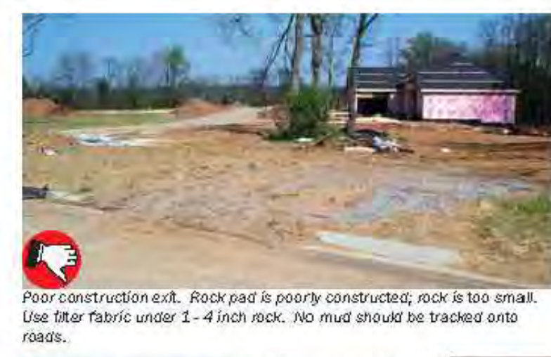
Poor construction exit. Rock pad is poorly constructed; rock is too small. Use filter fabric under 1-4 inch rock. No mud should be tracked onto roads.
