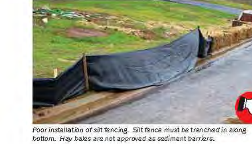
Poor installation of silt fencing. Silt fence must be trenched in along bottom. Hay bales are not approved as sediment barriers.
