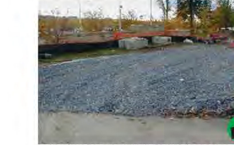
Good stabilized construction entrance. Adequate width to accommodate construction traffic and prevent mud tracking onto neighboring streets. Ensure that the pad is 8 inches deep and 40 feet long. Stabilize Construction Entrance
