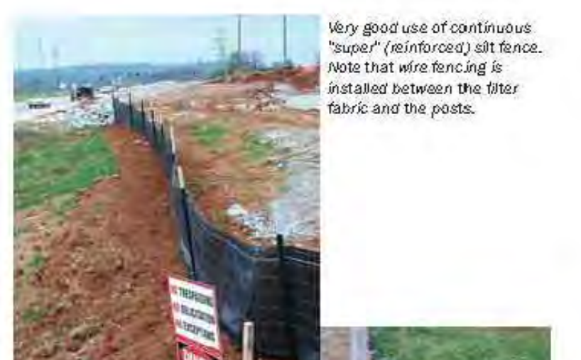
Very good use of continuous "super" (reinforced) silt fence. Note that wire fencing is installed between the filter fabric and the posts.
