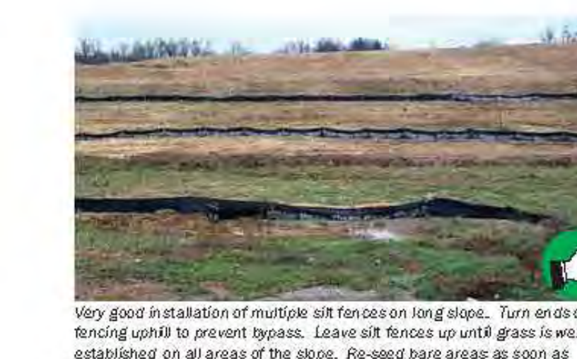
Very good installation of multiple silt fences on long slope. Turn ends of fencing uphill to prevent bypass. Leave silt fences up until grass is well established on all areas of the slope. Re-seed bare areas as soon as possible. Remove or spread accumulated sediment and remove silt fence after all grass is up.
