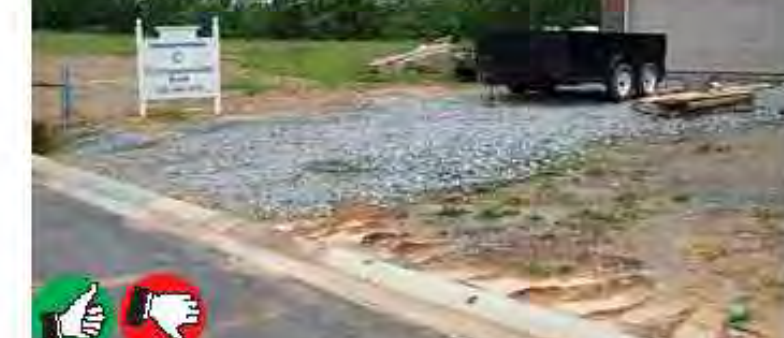
Rock sizing and placement look OK for residential site, and very little mud appears on the road. The pad should be at least 8 inches thick and 12 feet wide. Ensure that pad is used as the entrance and exit points - note track marks near curb. Entire area needs seed and mulch.
