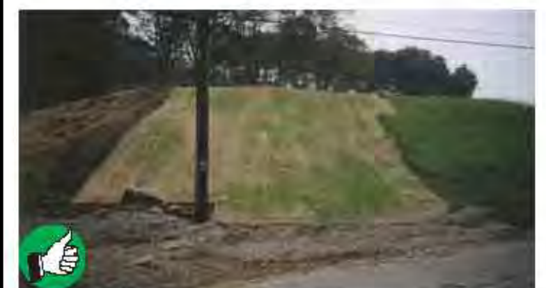
Excellent stabilization of large slopes to limit the area of disturbance. Make sure to install erosion control matting within 48 hours of grading to ensure good contact between soil and mat.
