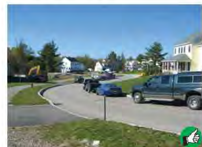
This residential subdivision is being constructed in phases. To limit the total disturbance area, only a few home sites are under construction at one time.
