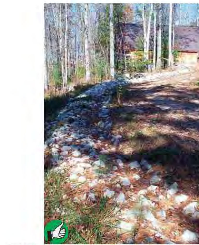
Good installation of rock-lined berm to divert rain runoff around residential construction site on steep slope near a river. Diversion ditches can be lined with grass if channel slopes are 5% or less, and with 4 inch stone if they are steeper.
