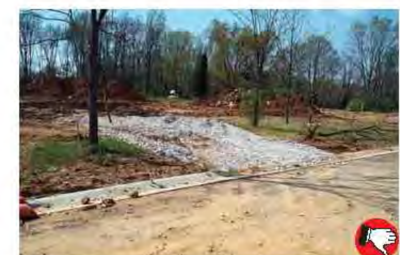
Rock pad was installed properly with right sized rock, but lack of filter fabric underliner is causing rock to spread and sink into the soil. Note tracking of mud onto road. Mud tracked on roadways violates the permit requirements and is a potential legal liability.
