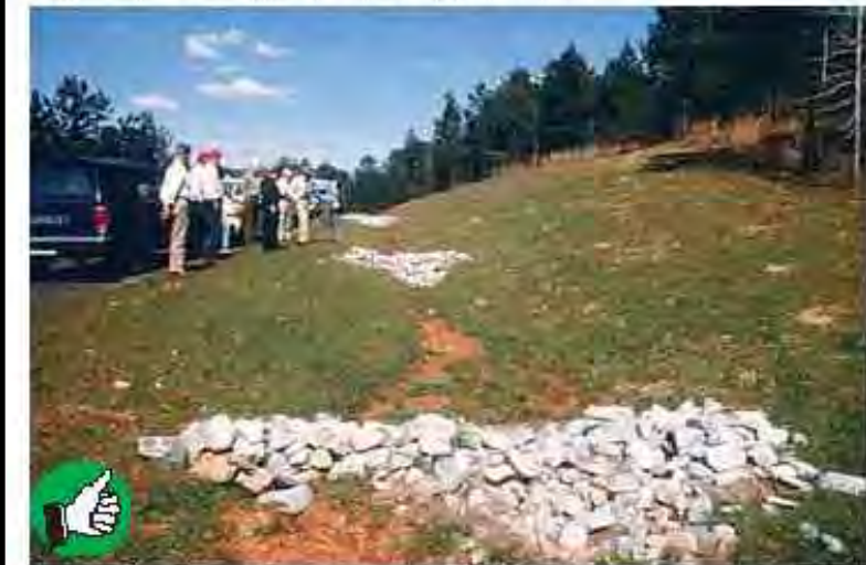
Good installation of temporary rock check dams. The check dams should extend up the sides of the banks. Midline section should be lower than the sides. Clean out sediment as it accumulates. Remove check dams after site and channel are stabilized with vegetation.
