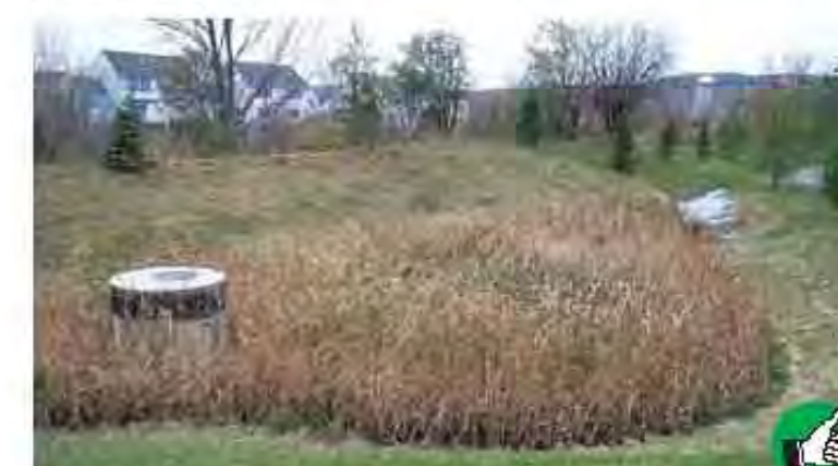
Install all permanent stormwater treatment practices before constructing any impervious surfaces on site. This stormwater wetland treats stormwater runoff from the adjacent parking lot.
