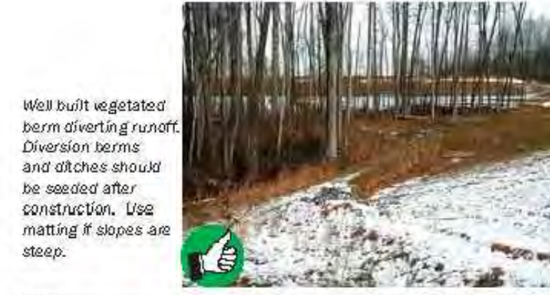
Well built vegetated berm diverting runoff. Diversion berms and ditches should be seeded after construction. Use matting if slopes are steep.
