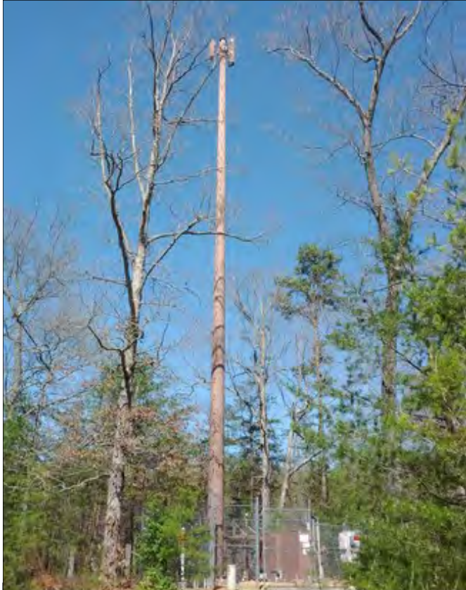
Narrow profile monopole towers such as this one tend to be less visually intrusive than larger lattice towers and towers with widely spaced arrays of antennas. “Stealth” towers designed to appear as trees or other landscape features can be effective, but only if they appear as natural parts of their surroundings.
