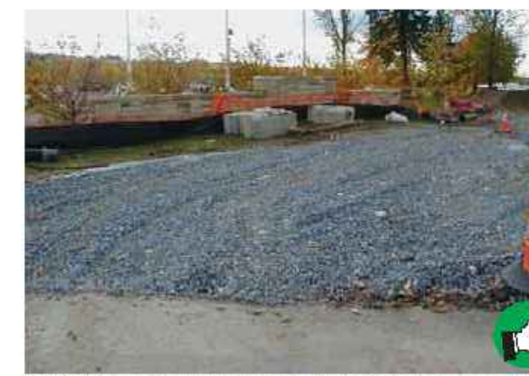
Good stabilized construction entrance. Adequate width to accommodate construction traffic and prevent mud tracking onto neighboring streets. Ensure that the pad is 8 inches deep and 40 feet long. Stabilize Construction Entrance
