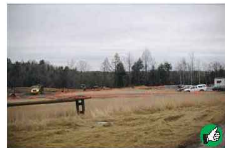
Properly placed barrier tape marks the boundaries and limits of construction on this site.
