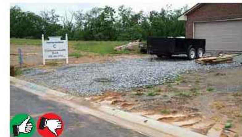
Rock sizing and placement look OK for residential site, and very little mud appears on the road. The pad should be at least 8 inches thick and 12 feet wide. Ensure that pad is used as the entrance and exit points - note track marks near curb. Entire area needs seed and mulch.
