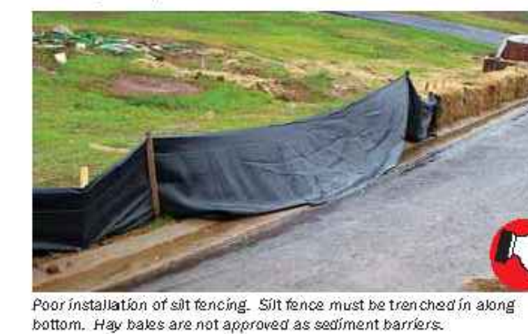
Poor installation of silt fencing. Silt fence must be trenched in along bottom. Hay bales are not approved as sediment barriers.
