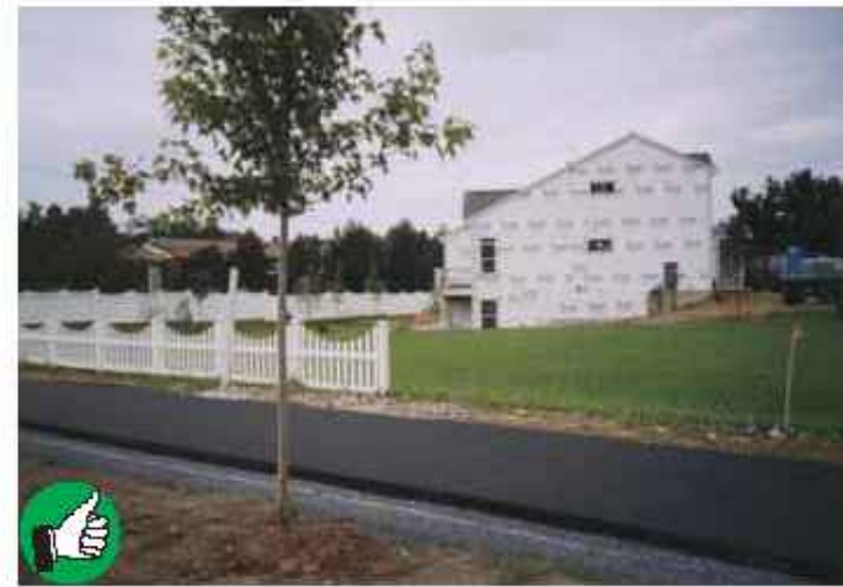
Lawn is fully established before construction is completed at this home site.
