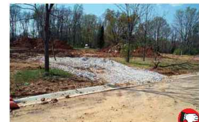
Rock pad is installed properly with right sized rock, but lack of filter fabric underlayment is causing rock to spread and sink into the soil. Note tracking of mud onto road. Mud tracked on roadways violates the permit requirements and is a potential legal liability.
