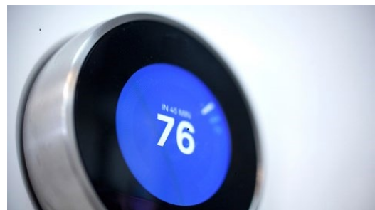
Smart thermostats provide customers with value on multiple fronts: easy time-of-day scheduling for desired temperatures and ensuring cost-savings during unoccupied periods.
