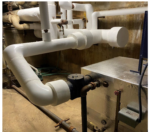
Installing mechanical insulation on steam pipes can result in a dramatic decrease in heat loss.
