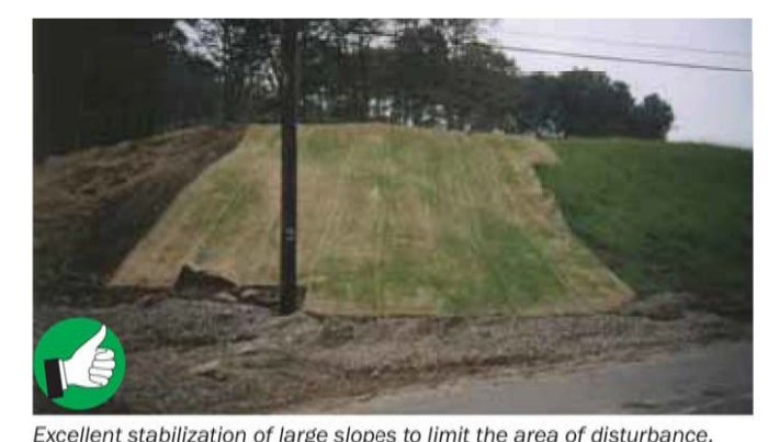
Excellent stabilization of large slopes to limit the area of disturbance. Make sure to install erosion control matting within 48 hours of grading to ensure good contact between soil and mat.
