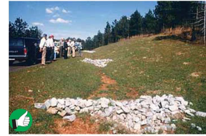
Good installation of temporary rock check dams. The check dams should extend up the sides of the banks. Middle section should be lower than the sides. Clean out sediment as it accumulates. Remove check dams after site and channel are stabilized with vegetation.
