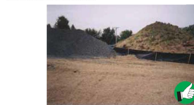
Excellent application of hay mulch. Good mulch cover and sediment barrier around soil stockpile.
