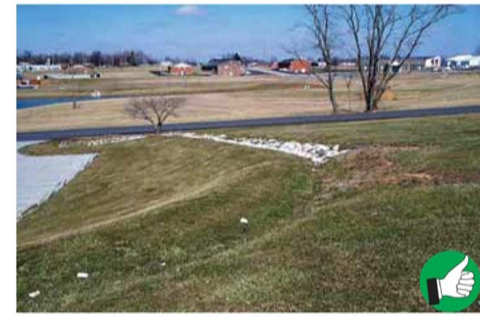
Good construction, seeding, and stabilization of diversion berm. Note that diversion ditch is lined with grass on flatter part of slope, and with rock on steeper part.
