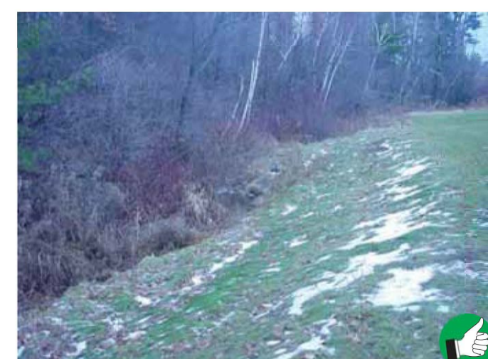
Stabilization and seeding of slopes before winter will reduce or eliminate erosion in the spring. The grass on this slope is holding the soil in place and promoting infiltration of the melting snow.
