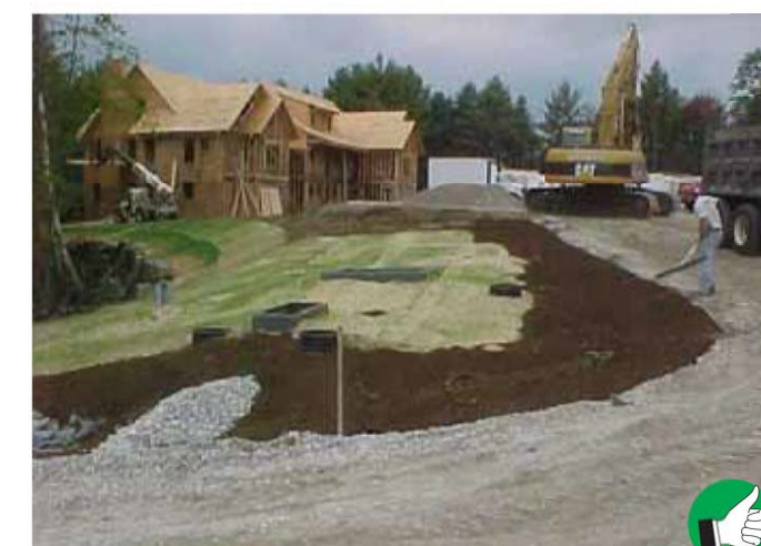
Within 48 hours of final grading, erosion control matting and mulch have been applied.
