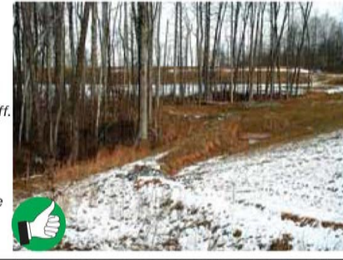
Well built vegetated berm diverting runoff. Diversion berms and ditches should be seeded after construction. Use matting if slopes are steep.
