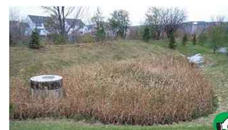
Install all permanent stormwater treatment practices before constructing any impervious surfaces on site. This stormwater wetland treats stormwater runoff from the adjacent parking lot.
