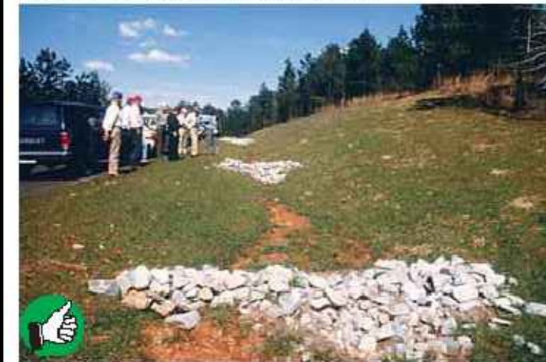
Good installation of temporary rock check dams. The check dams should extend up the sides of the banks. Midline section should be lower than the sides. Clean out sediment as it accumulates. Remove check dams after site and channel are stabilized with vegetation.
