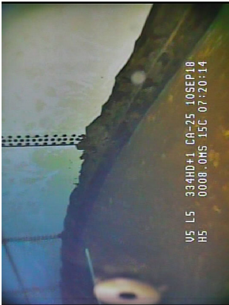
Interior CIM perimeter seal
