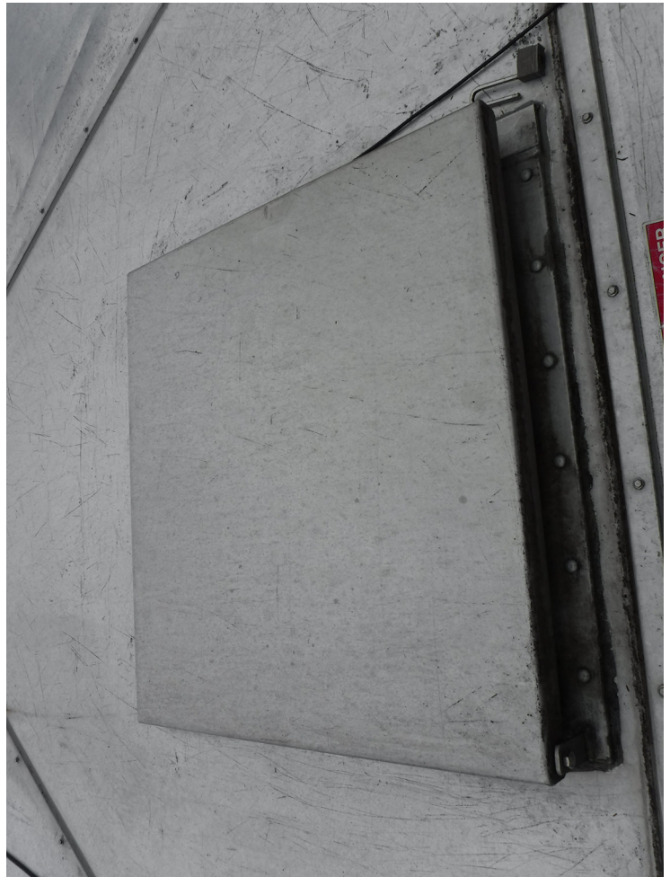
Roof man way hatch
