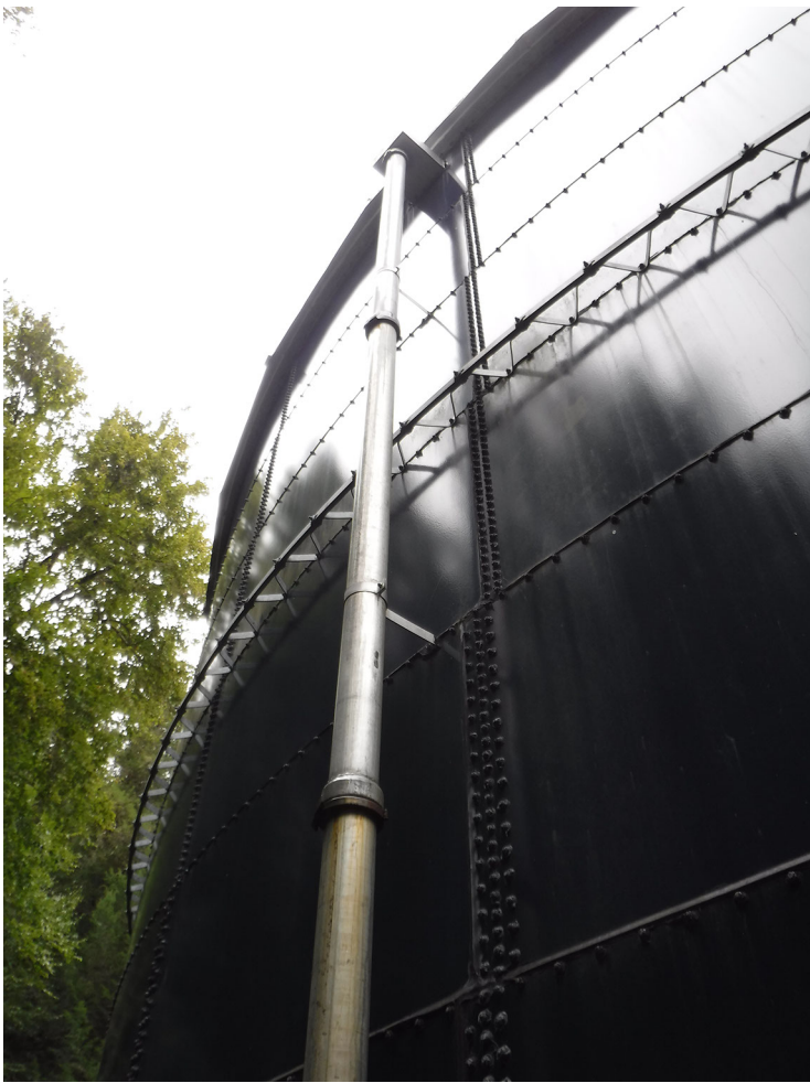
Overflow pipe and weir box
