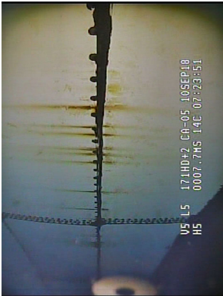
Interior horizontal seam corrosion (2)
