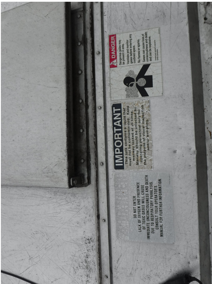
Roof safety decals
