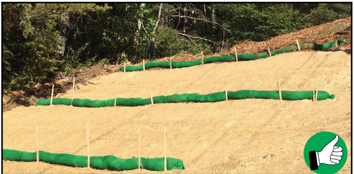
Good use of filter socks along a slope to slow runoff velocity.
