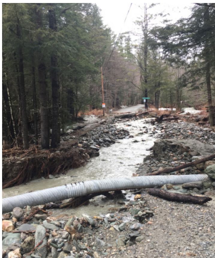
Flood Damage of the Lilliesville Road Bridge in Stockbridge in April 2019 | Source: TRORC Staff
