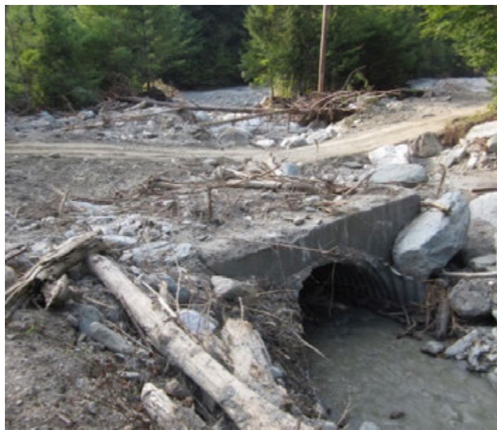
Severely Damaged Culvert, Stockbridge
