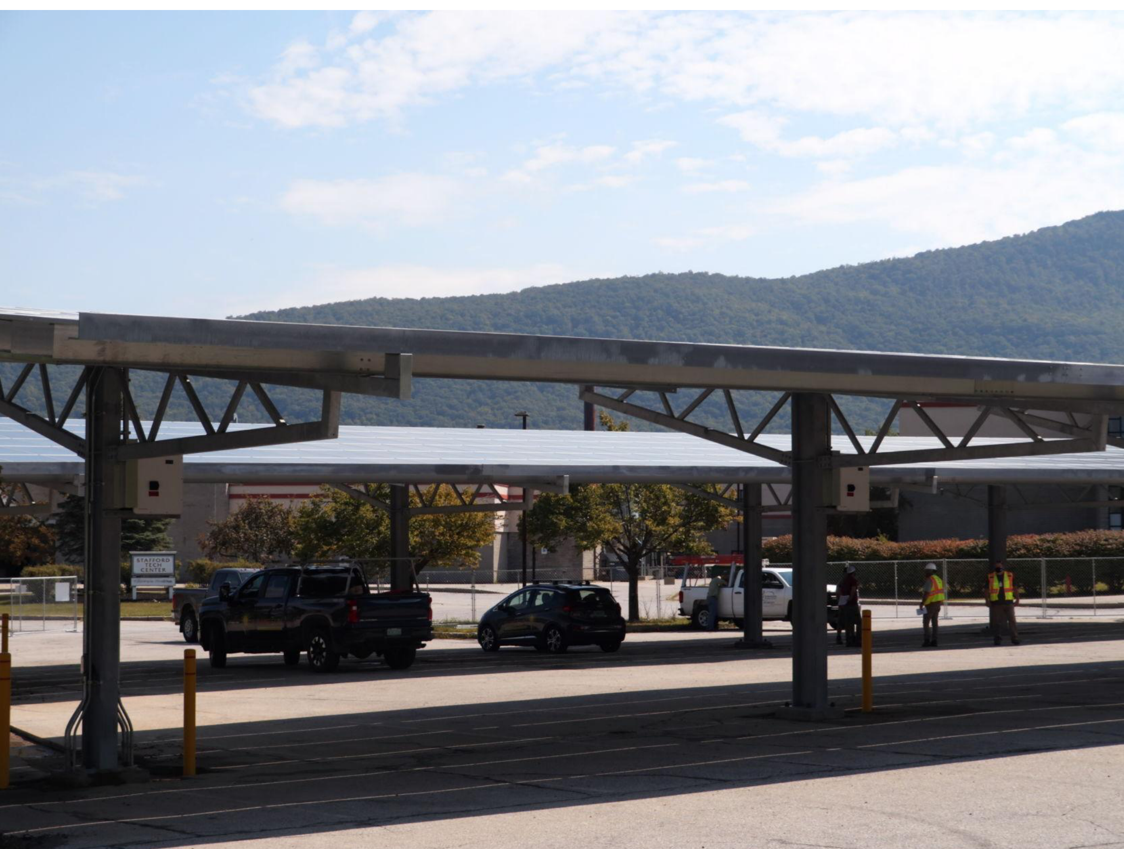
The solar canopy at Rutland High School. Jim Sabataso / Staff Photo
