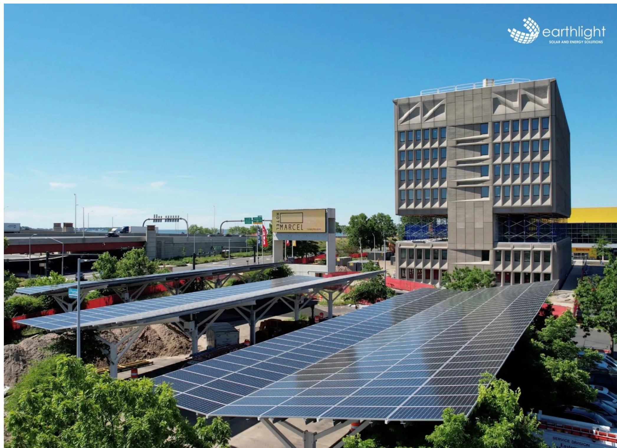
A solar canopy at the Hotel Marcel in New Haven. Credit: Earthlight Technologies / Courtesy
