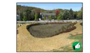
Infiltrating stormwater practices such as this bioretention system should be kept offline until the drainage area has been fully stabilized.
