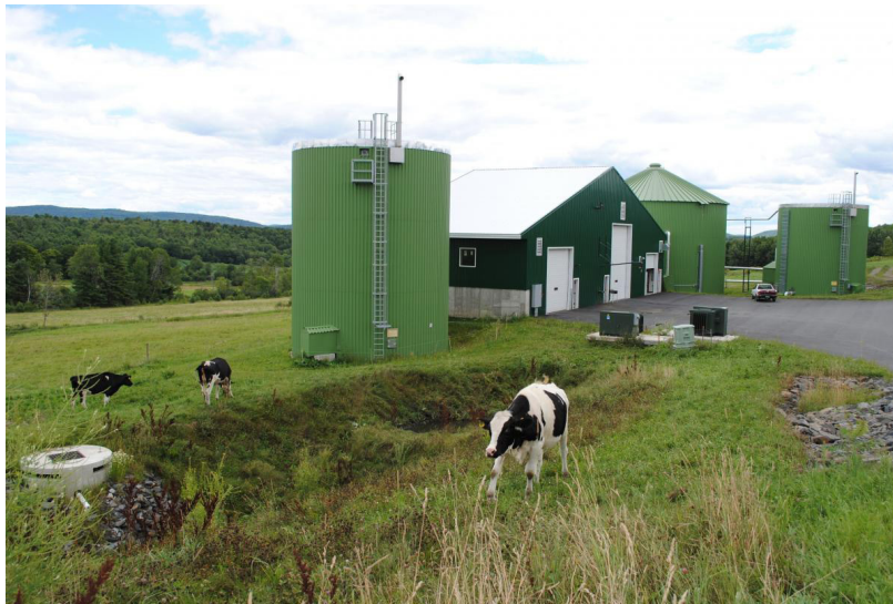
Anaerobic Digester, Vermont Technical College
