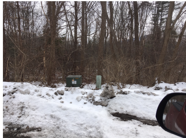
Buried Electrical Equipment End of Russett Drive
