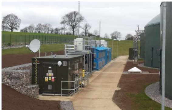
DMT Carborex ® MS in the UK, 1500 SCFM raw biogas upgrading for gas grid injection
