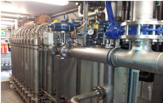
DMT Carborex ® MS in the UK, 500 SCFM raw biogas upgrading for grid injection
