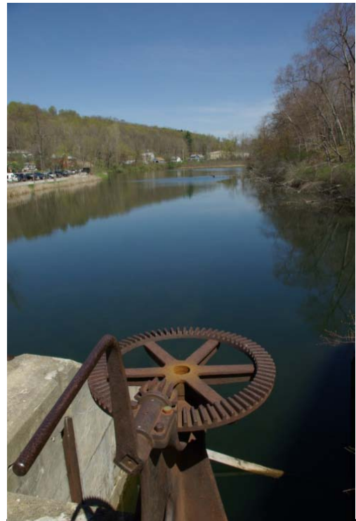
Penstock controls at one of four dams on Paran Creek in North Bennington. Other existing dam sites that can be redeveloped to produce electricity include the dam at Lake Paran, the Vermont Tissue dam on the Walloomsac River in Bennington, the dam at the old tannery site on the Hoosick River in Pownal, and dams on the east and west branches of the Batten Kill in Manchester.
