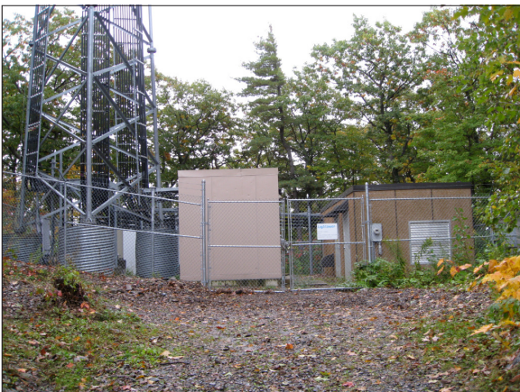
Existing cell tower equipment on Georgia Mountain, Milton
